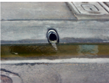
Backyard water draining to street.
